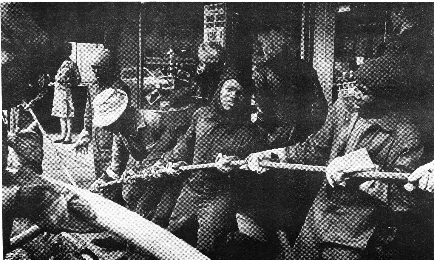
Black workers installing cable in Johannesburg. These workers still do not have basic trade union rights.
