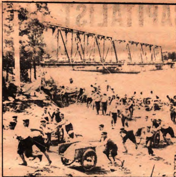
During the recent Tangshan earthquake in China, People's Liberation Army fighters worked day and night to repair the railway
