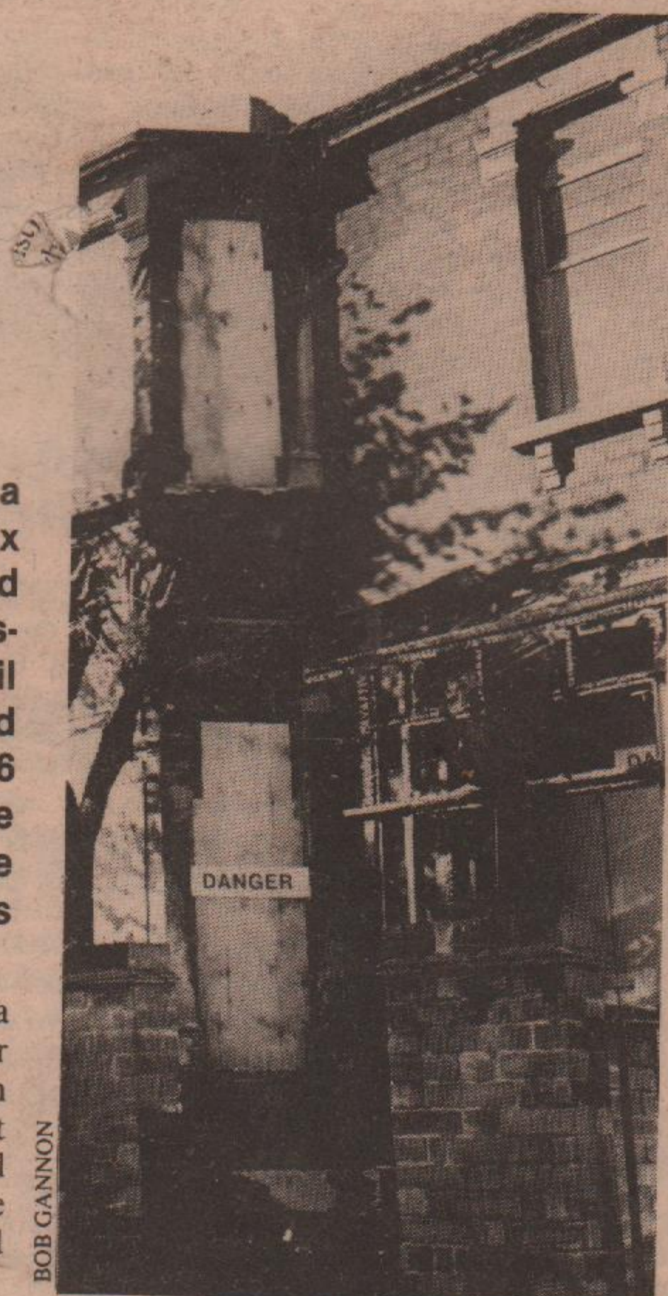
The burnt out shell of the fire bombed house
