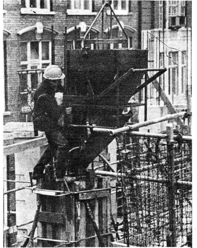
Hazards of working on a building site are worsened by a lack of safety equipment photo: Andrew Wiard (Report) (II)
