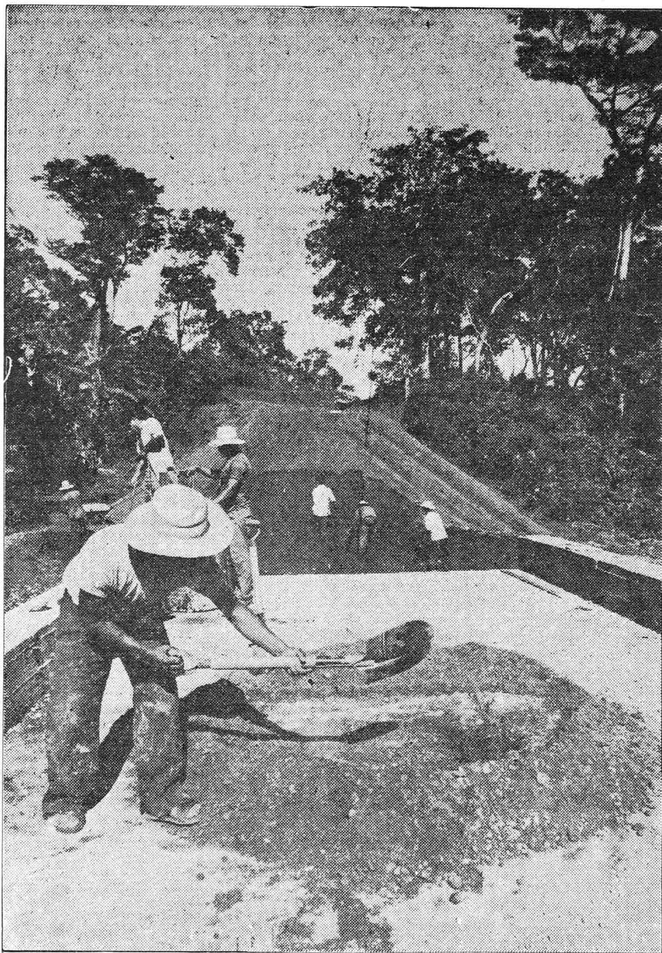
Building a road in Veracruz state. Of Mexico's 18 million workers, 45% do not have a steady full-time job.
