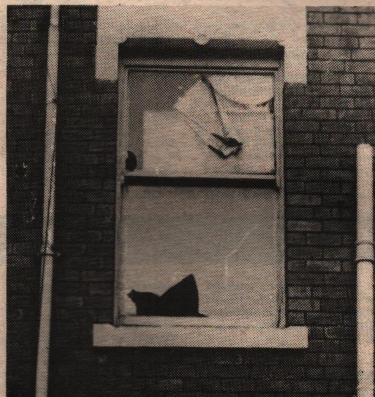
... and a window broken by a Nazi brick.
