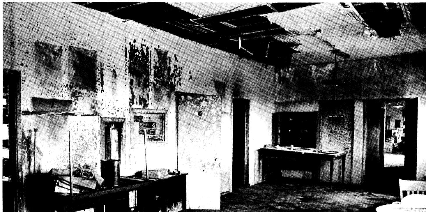
Photos indicate arson damage to SWP hall
