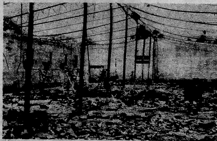
Somoza and his henchmen wrecked the country before fleeing into exile. Above, Nicaragua's largest sugar refinery after being destroyed by Somoza's bombs.
