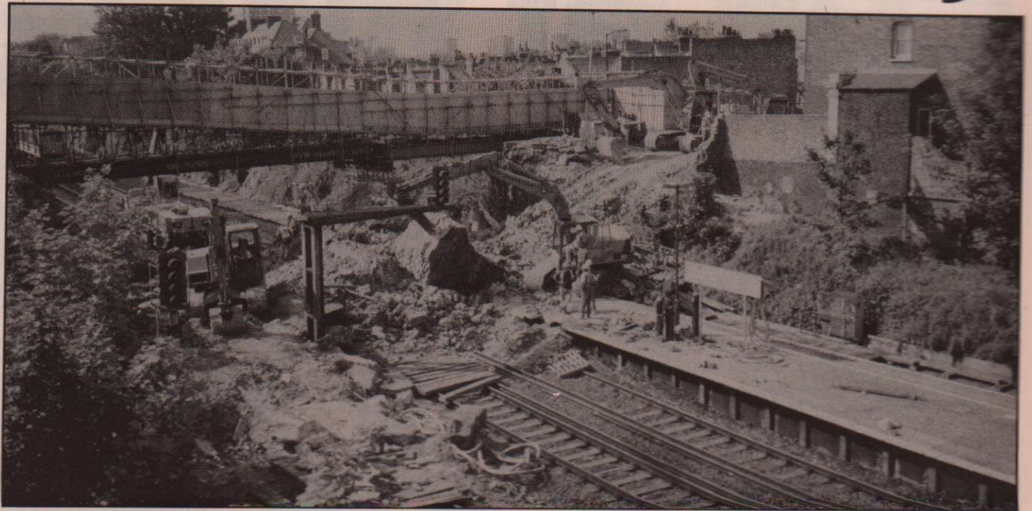
The St John's station bridge, June 1992: Two men — Nicholas Scott and Frank Warren — were killed and five others injured
