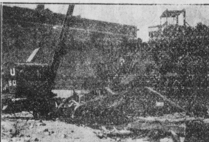
Two workers were killed and one is in the hospital in a serious condition when a crane fell on a Tenth Avenue construction job. The company is trying to saddle the blame on the workers. Photo taken yesterday by Film and Photo League shows the wreckage.
