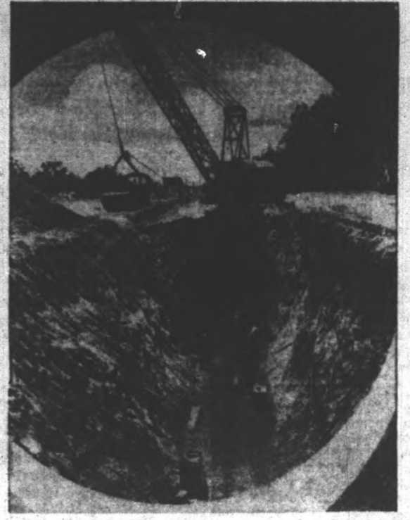
Thousands of workers are being kept busy on this new 242-mile pipeline that will carry the waters of the Colorado River to Los Angeles and other west coast cities. The concrete pipe will be from 10 to 12 feet in diameter—and that means lots and lots of water.
