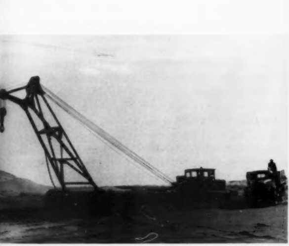
TURKMENIA is tapping its rich natural resources. Work in progress at the new oil fields recently discovered at Katur Tep.
