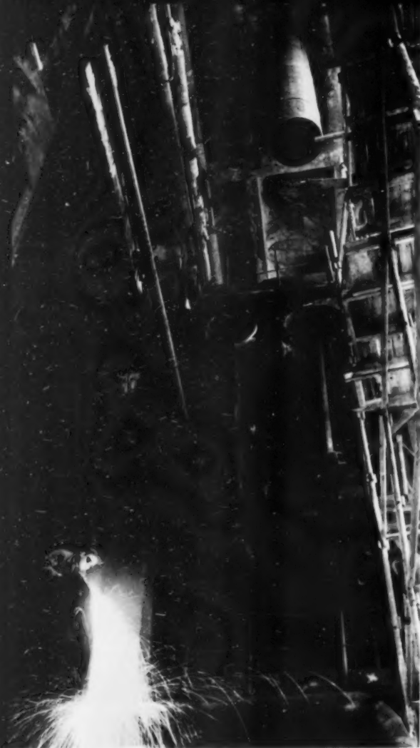
Alexander Kuznetsov is cutting up these outmoded gas generators that he helped assemble 20 years ago.
