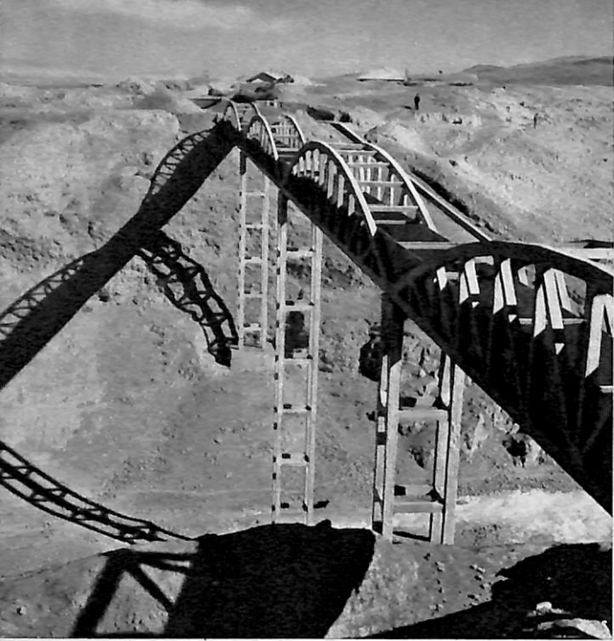
An aqueduct 92 metres long, part of the irrigation project being constructed in Tungteh County, Hainan Tibetan Autonomous Chou, to transform the Meilitan grassland.
