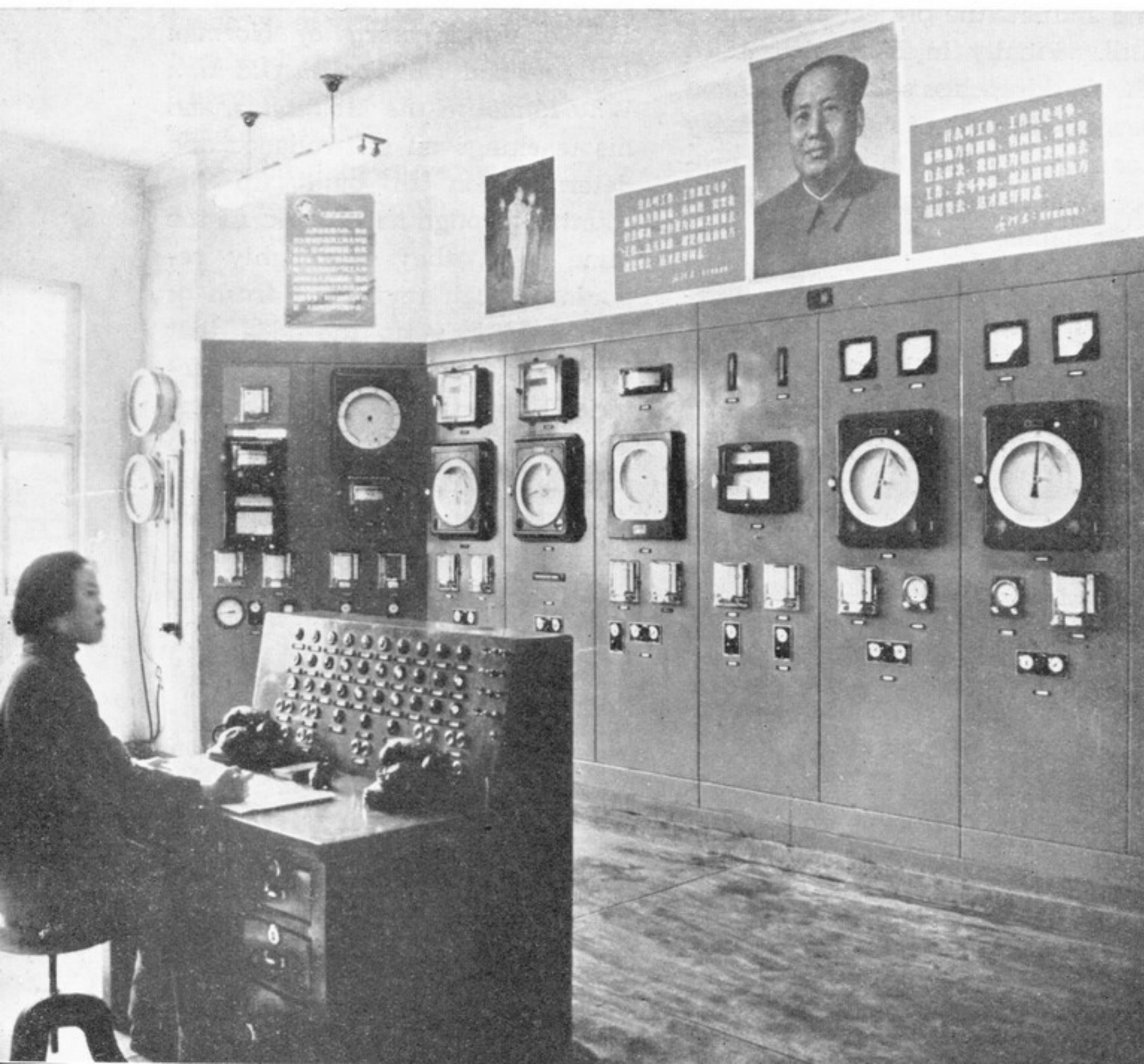
Automatic control board of the urea section.
