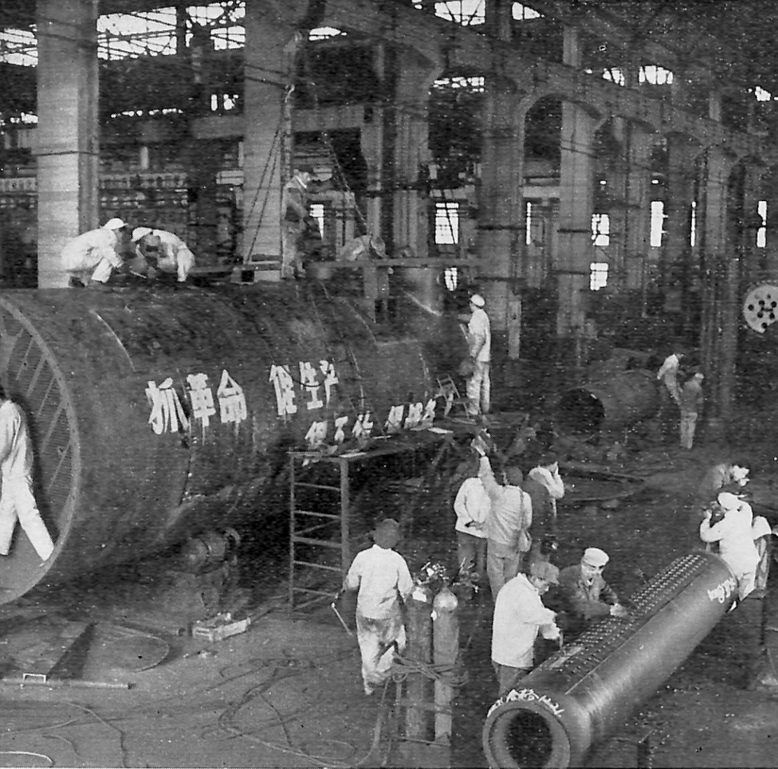
A shop in the boiler plant.
