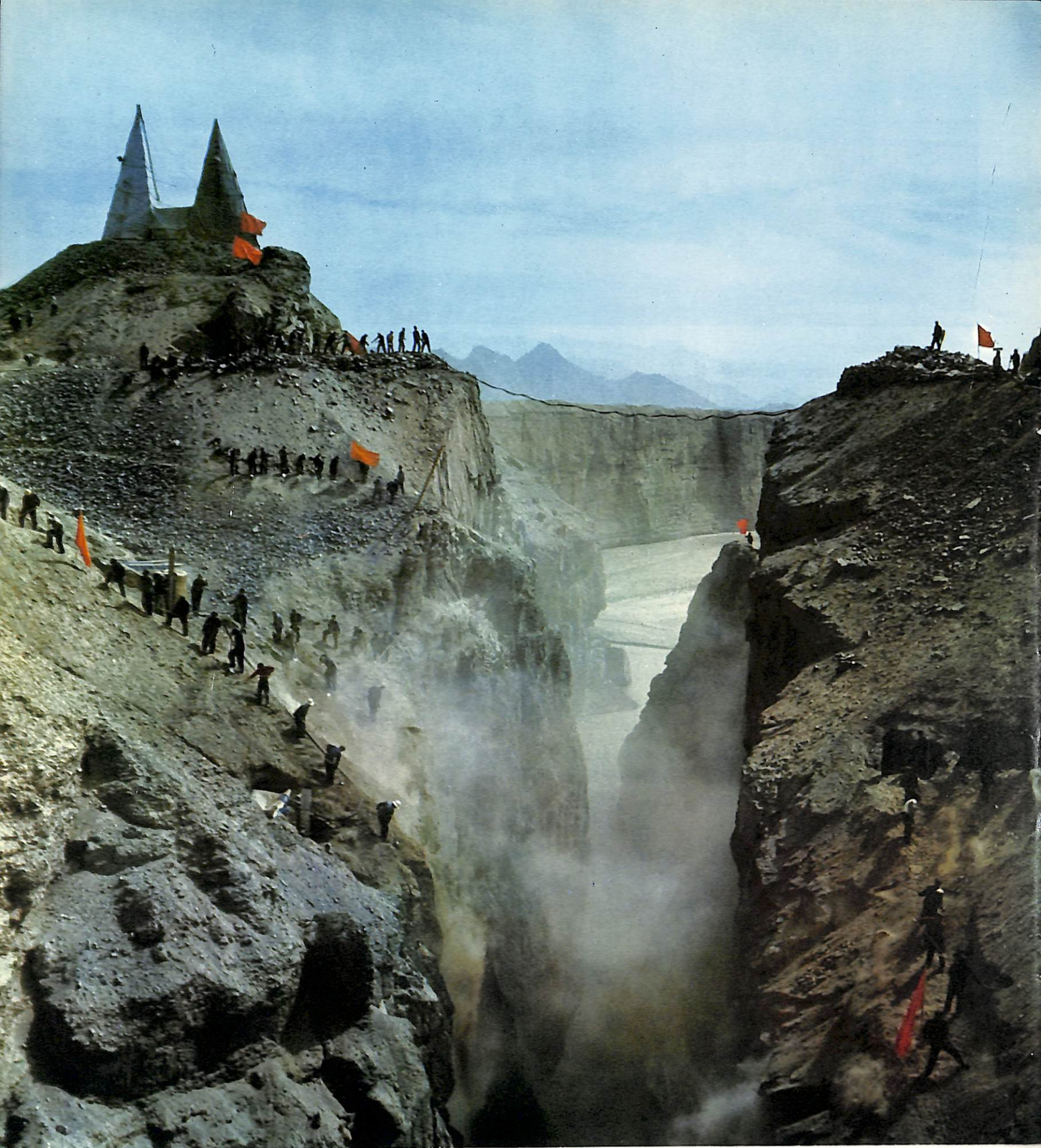
A view of the worksite of the hydropower station on the Karmo River.
