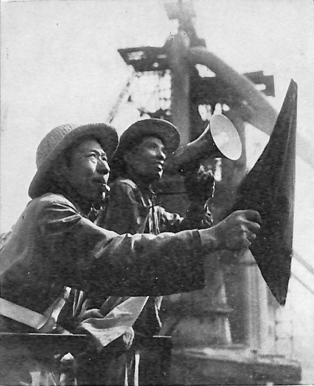
A signal is given directing an action in the enlargement of a furnace.
