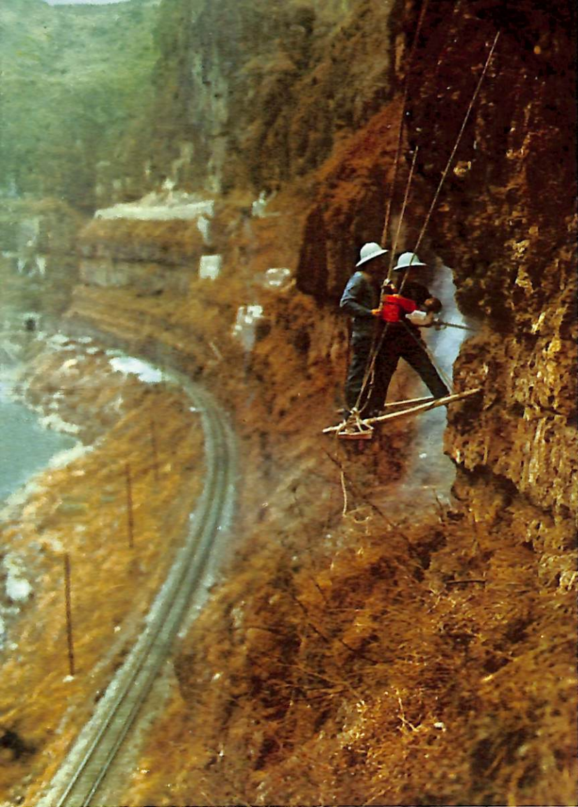
Maintenance men work the year round on cliffs along the line to prevent hazards and ensure safe rail traffic.
