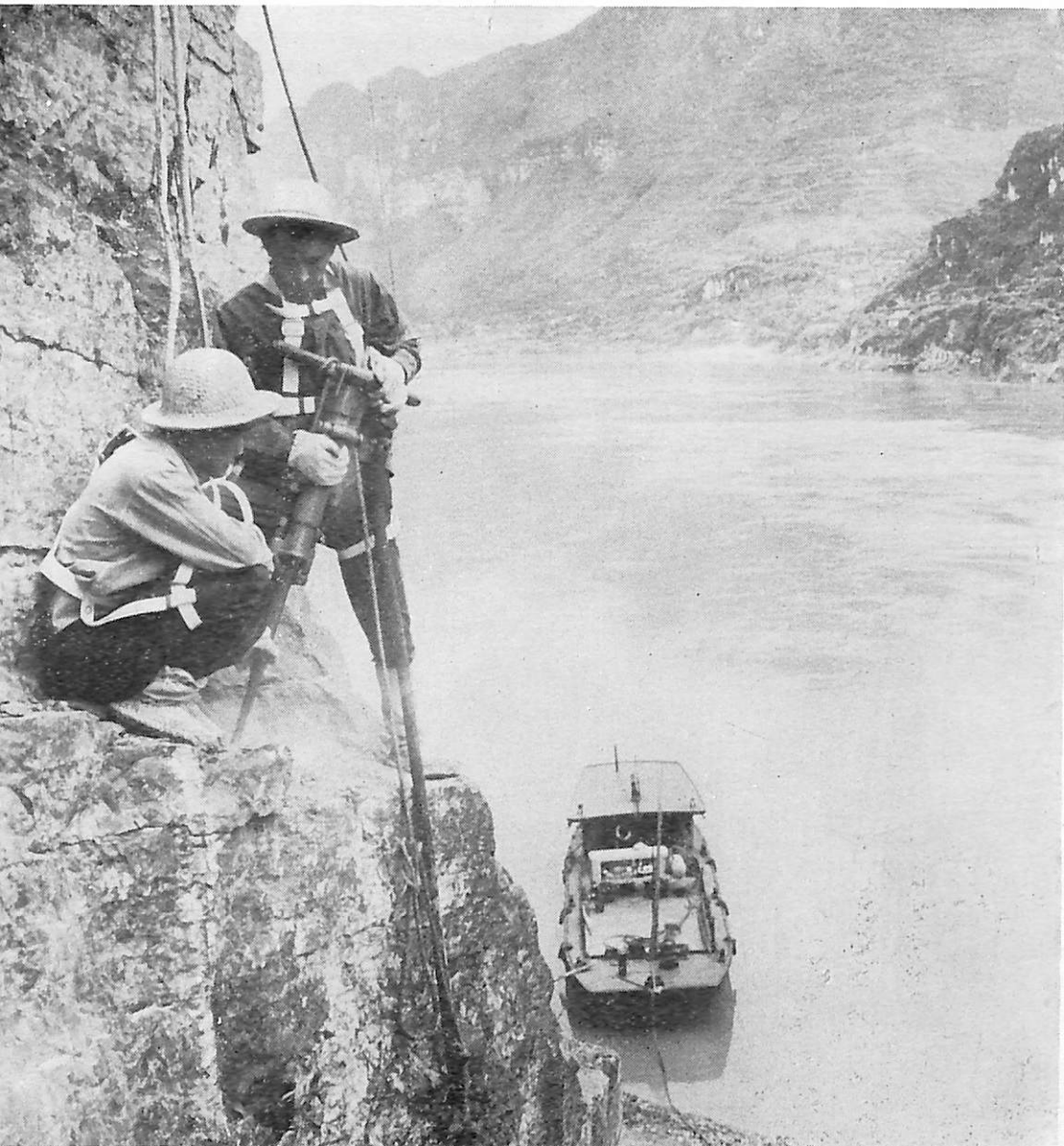
Workers remove a dangerous overhang to ensure safe passage in the channel.
