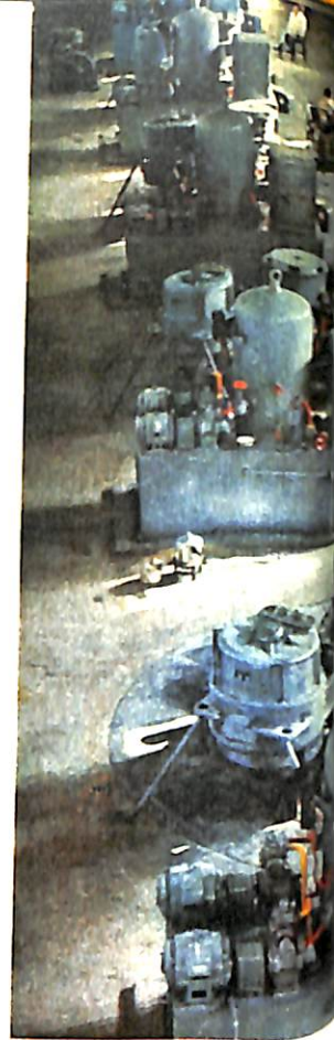
Generators in the Nyingchi industrial area.
