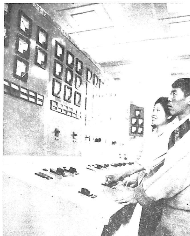
Control room in the "August 1" power station.
