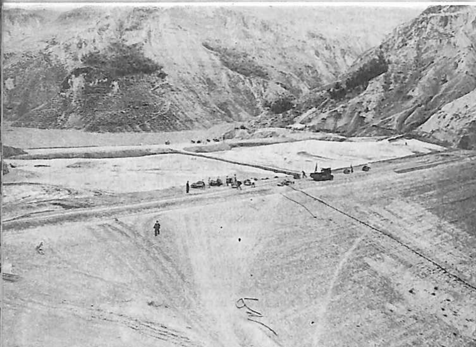
A flow of water carrying earth to build a dam, Zhangzishan commune, Zhongyang county, Shanxi province.
