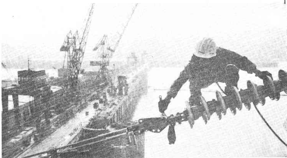
Perched precariously high above the river, an electrical worker checks connections on a generating unit of the second-channel power station.
