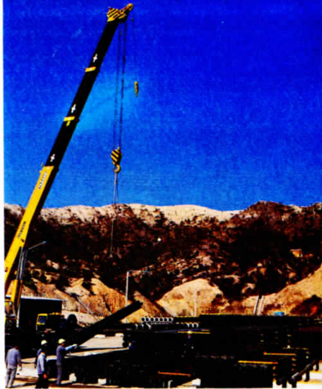
The transfer depot for casing pipes in Shenzhen's Shekou industrial area. Photo by Xu Jun
