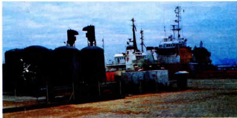
Modern equipment for blowing cement into an underwater well. Photo by Xue Chao
