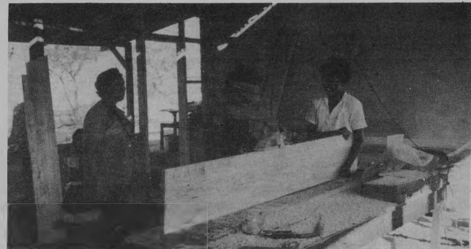
One of the biggest problems faced by Nicaragua is the shortage of materials but people are keen to build their new society. Here, local people are helping to build a new school for their children
