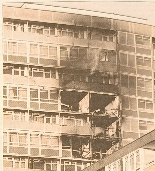
The shortage of adequate social housing means that many working class families end up in poorly-maintained tower blocks. Six people, including children, died in the fire that swept through this estate in Camberwell, south London in July 2009
