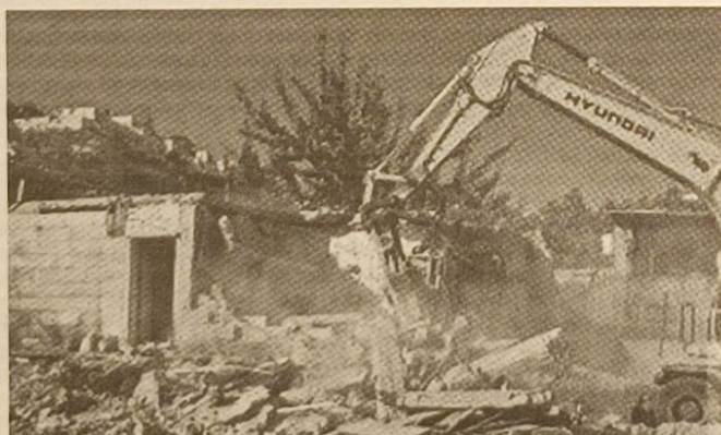
Demolition of a Palestinian home in the West Bank
